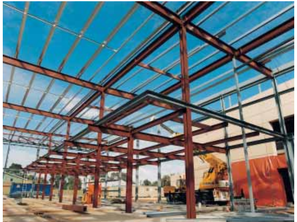
Significant time savings were achieved by the use of steel in the structure.
