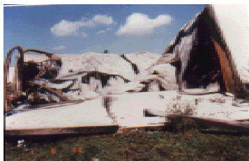
failure of connections causing external wall panels to collapse outwards during fire
