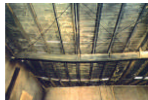
steel roof after fire
