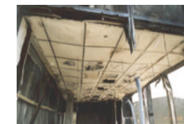
Ceiling after test
