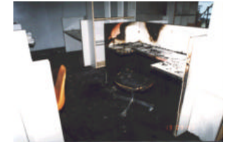
Extent of damage after Test 2
