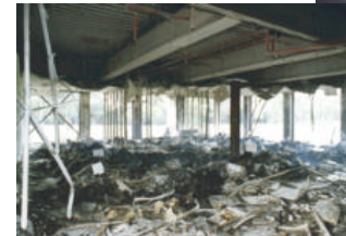
Extent of material consumed after fire
