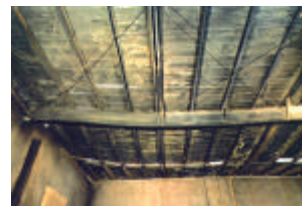
steel roof after fire
