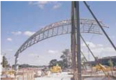
Top: Erection of the barrel vaults along the length of the railway station.
