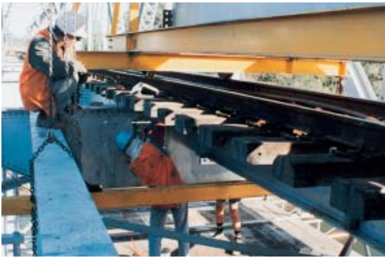
Figures 9 and 10. Removal of old, and installation of new beams at Boyne River bridge, showing underslung scaffold for safe working access.
