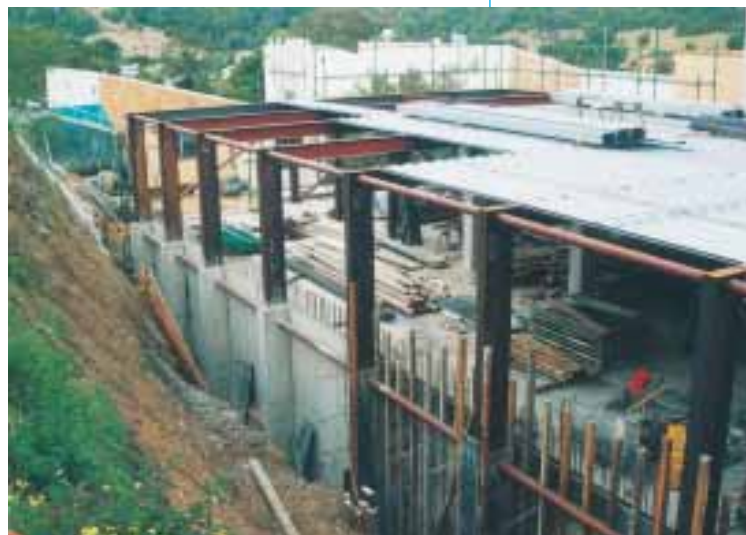
The steel frame serves as retaining wall on the deeply excavated site.
